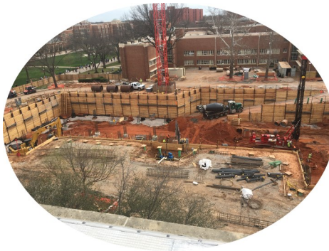
Future site of Lin Hall which is part of the Dodge Complex - Substantial Completion date July 2, 2018
